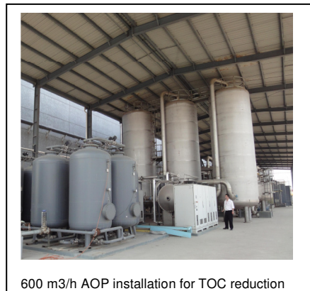
600 m3/h AOP installation for TOC reduction
