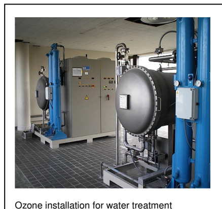
Ozone installation for water treatment
